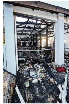
Completely destroyed: the garages where the fire broke out.
