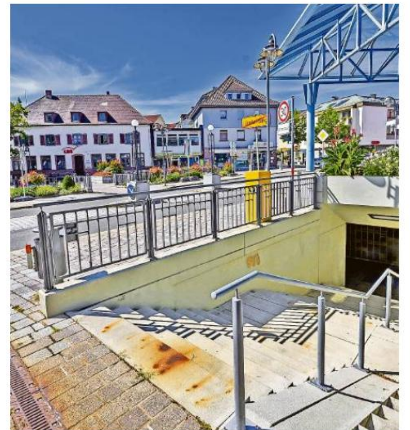
From above, the underpass at the market square in Birkenfeld appears gloomy. Parents find this section of the route to school is too scary for their children.
